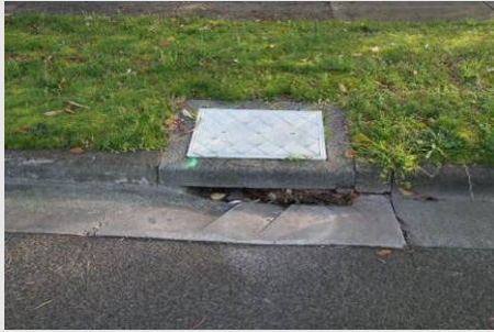
DE-001 Debris obstructing pit inlets
