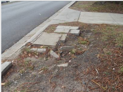
DE-007 Pit surrounds damaged to the extent that they are hazardous to road users/ pedestrians
